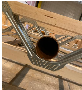
PD24: Piping and ventilation ducts
